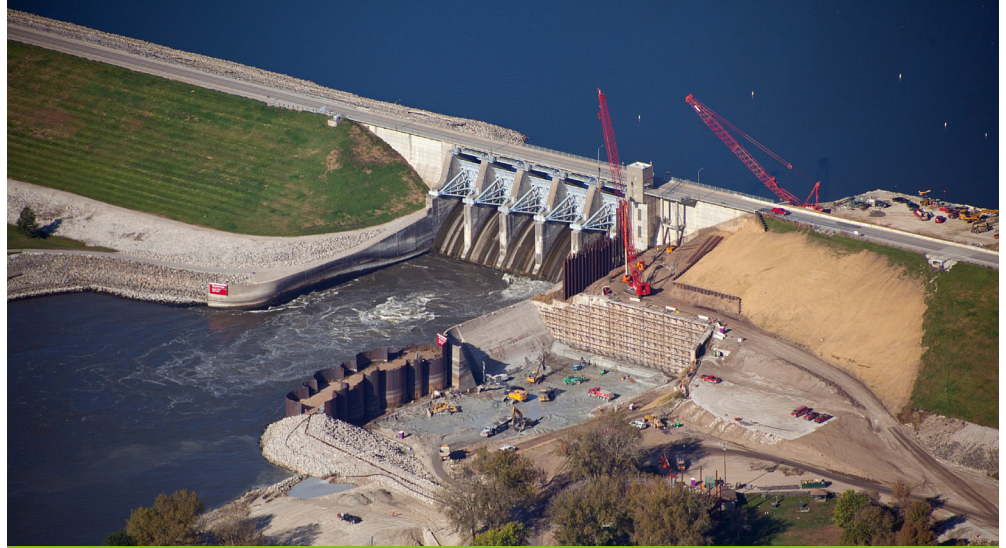
Red Rock Hydroelectric Project located just outside of Pella, Iowa, on the Lake Red Rock Dam. Photo credit Missouri River Energy Services.
